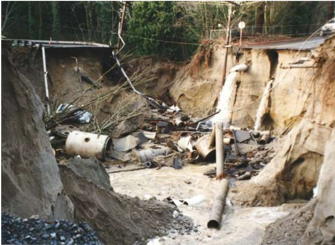
Photo 150 ~ On January 1, 1997, Shoreline suffered its first disaster - a major washout of NW 175th St. at 6th Ave NW. Due to excessive runoff created by an unusually heavy snowstorm and rapid melting, Boeing Creek jumped its culvert, and created Shoreline's "Little Grand Canyon," inconveniencing the neighborhood's residents for months. Note the car at far left lying down the embankment above large cement culvert pipe. Donated by Lynn Cheeney.
